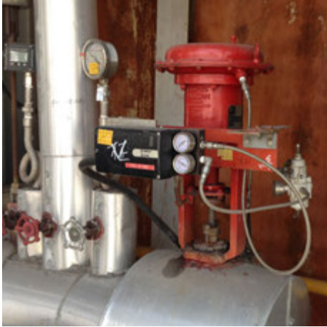
D20 installed on control valve
